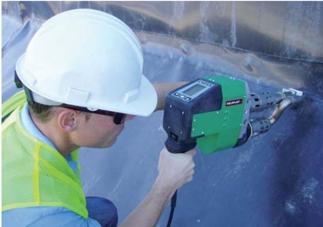
The WELDPLAST S4 whilst joining the plastic sealing tracks to the shore boarding.
